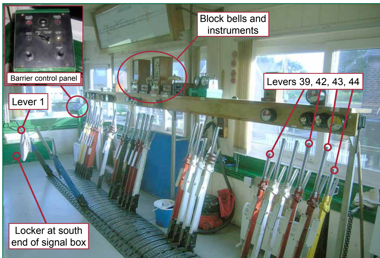
Figure 7: Signalling and level crossing controls in Moreton-on-Lugg signal box
