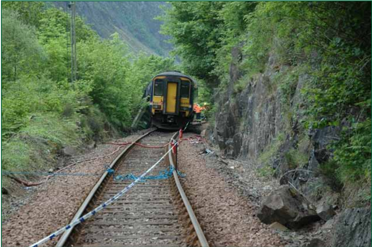
Figure 6: Exposed rock face area of the slope showing blocks
