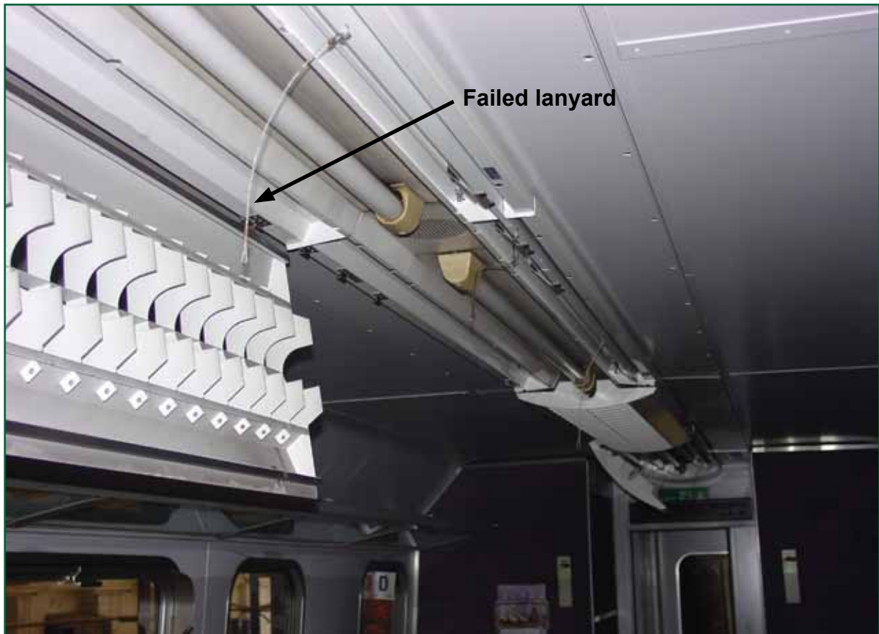
Figure 11: Lighting diffusers hanging down as a result of the collision
