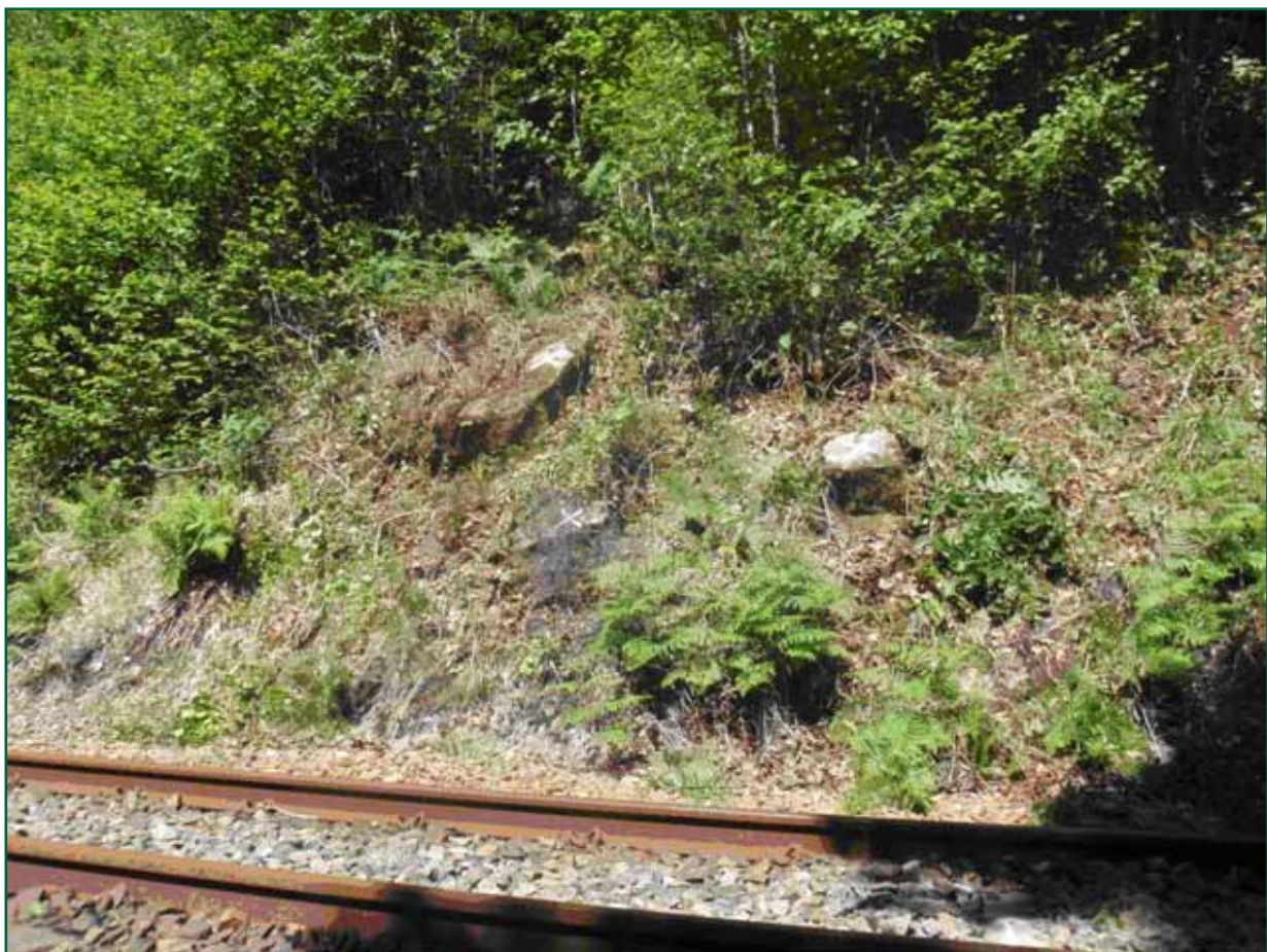
Figure 7: Area of soil slope containing isolated boulders (following post-accident de-vegetation) (image courtesy of Network Rail)
