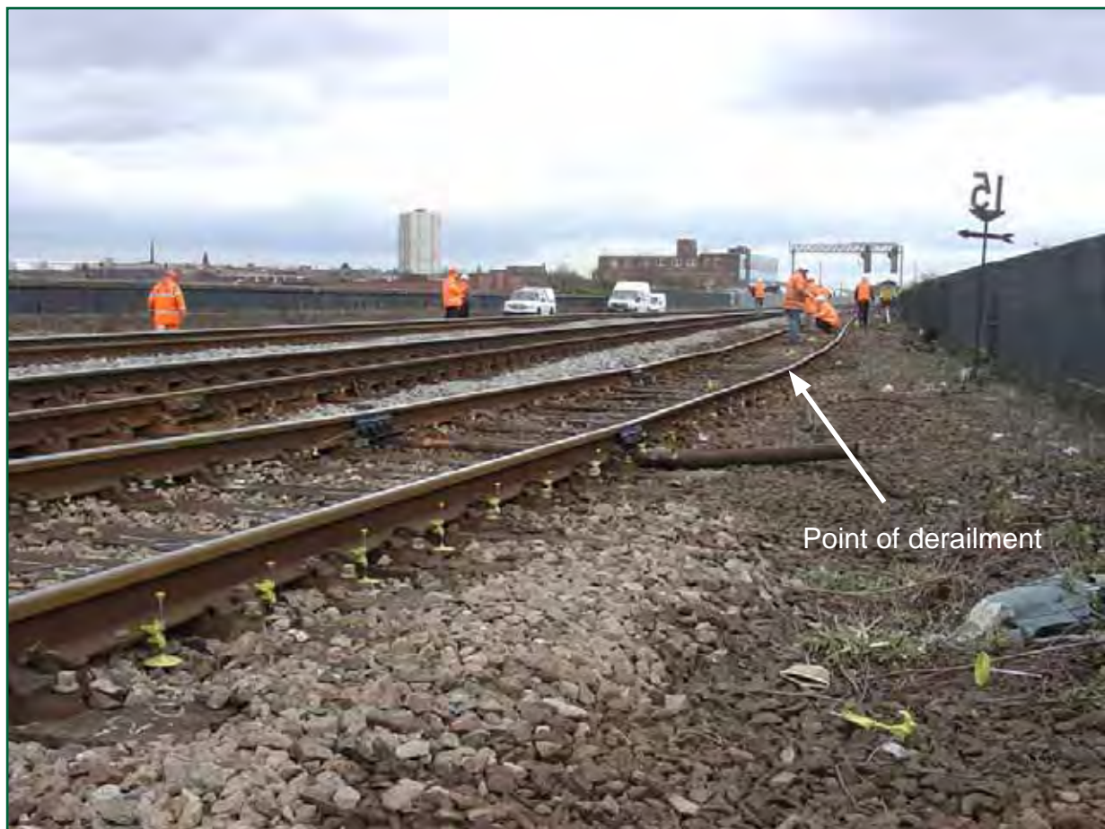
Figure 6: Track at the point of derailment
