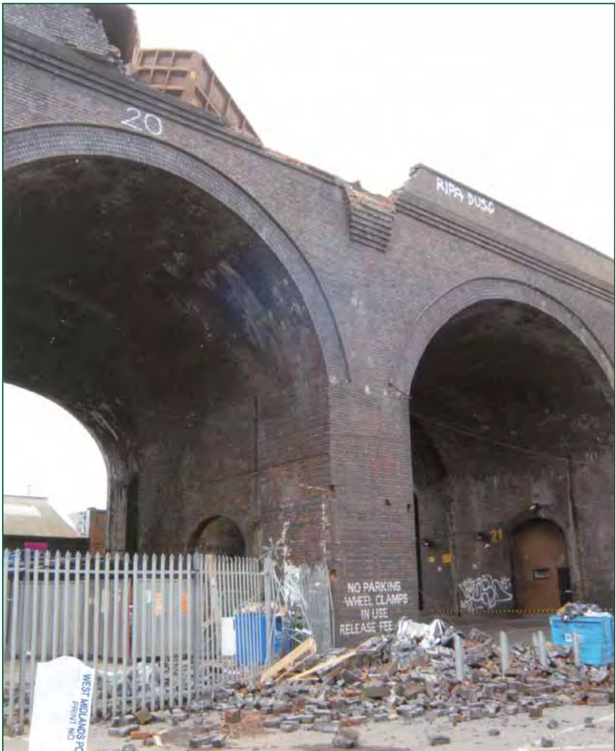
Figure 10: Fallen debris and damage to the parked car (image courtesy of West Midlands Police)
