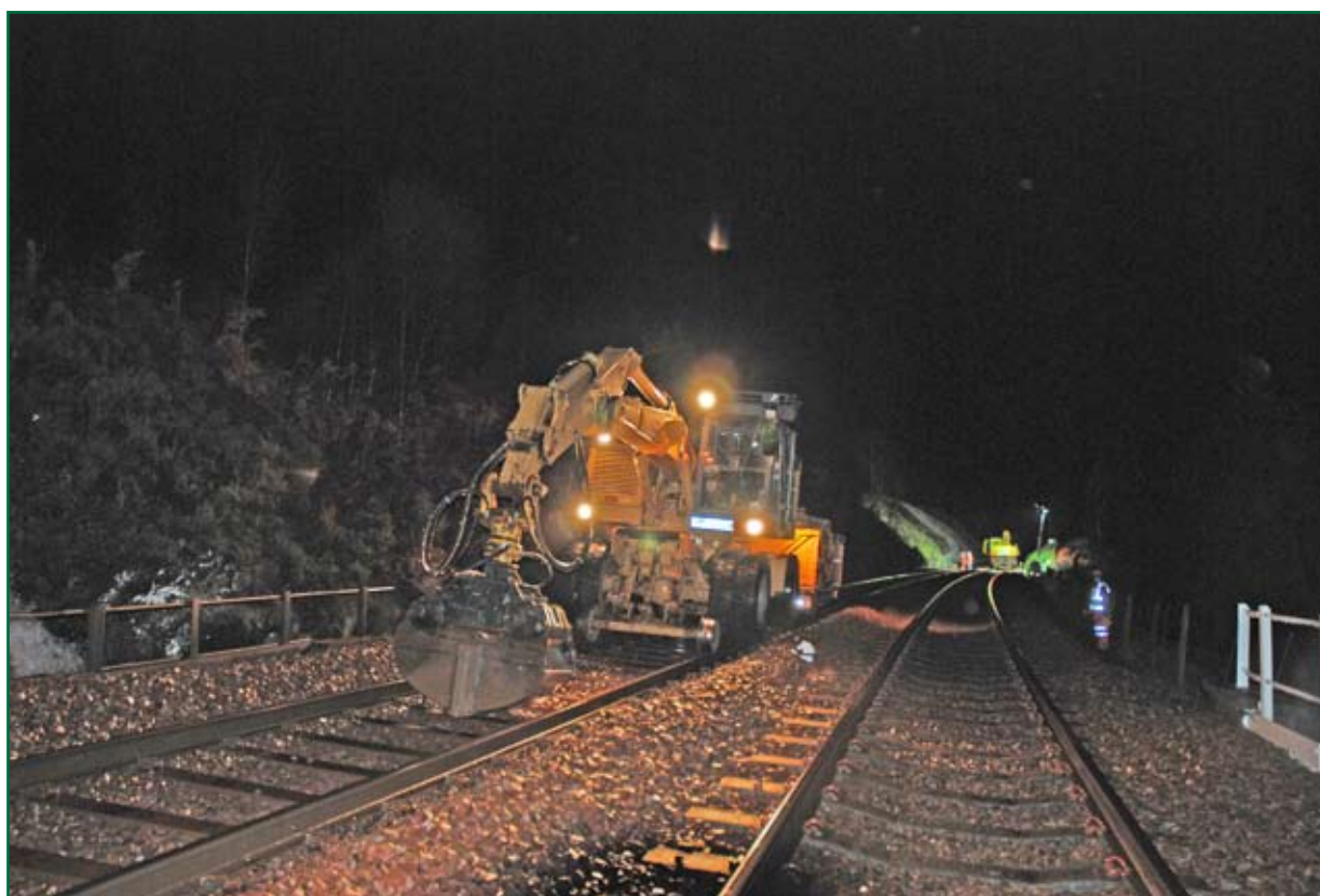
Figure 3: Colmar RRV and trailer immediately after incident (photo courtesy of Edmund Nuttall Ltd).
