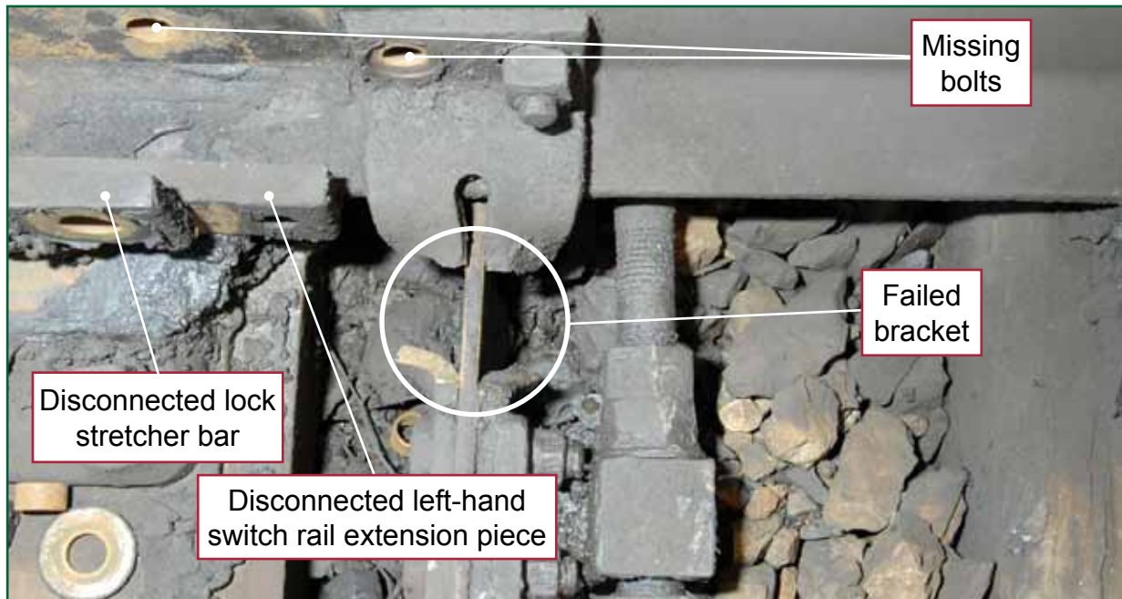
Figure 16: Failed bracket first permanent way stretcher bar
