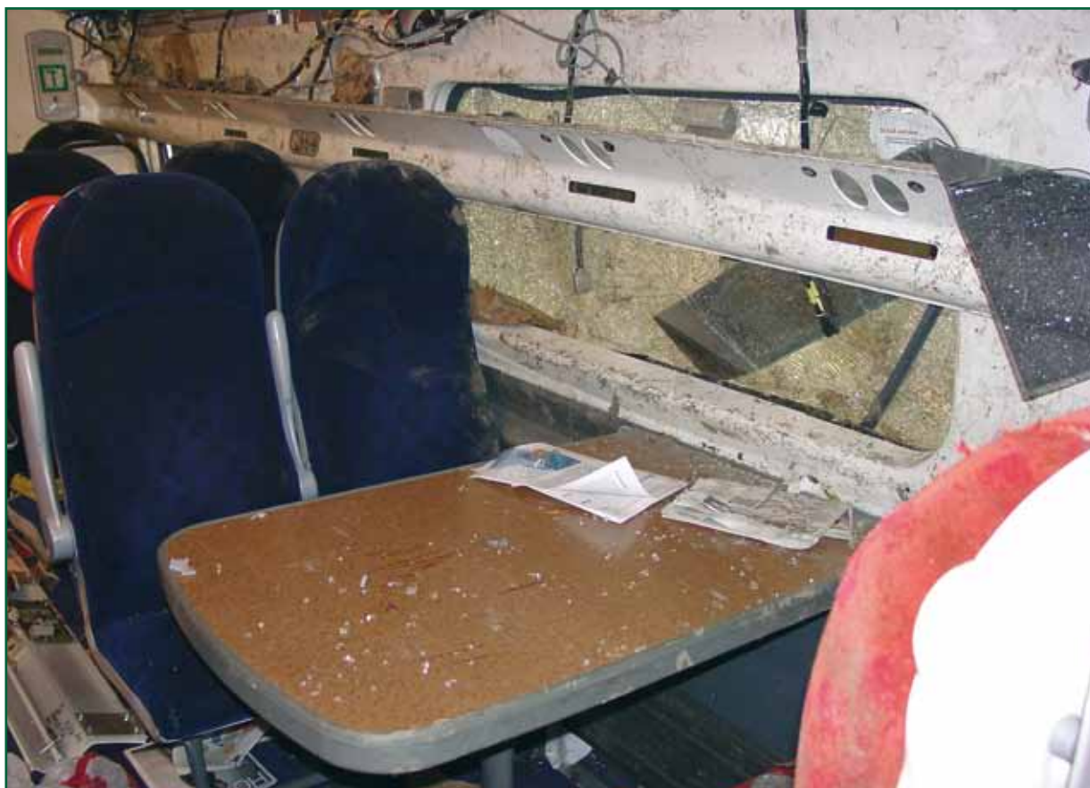
Figure 39: Detached reading light panels in the leading right-hand side of vehicle one
