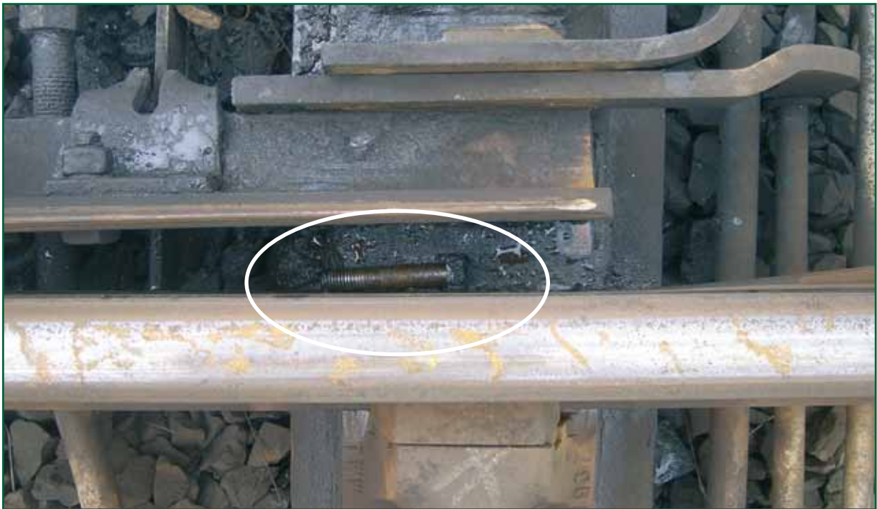
Figure 12: Lock stretcher bar bolt between left-hand switch and stock rail at toe
