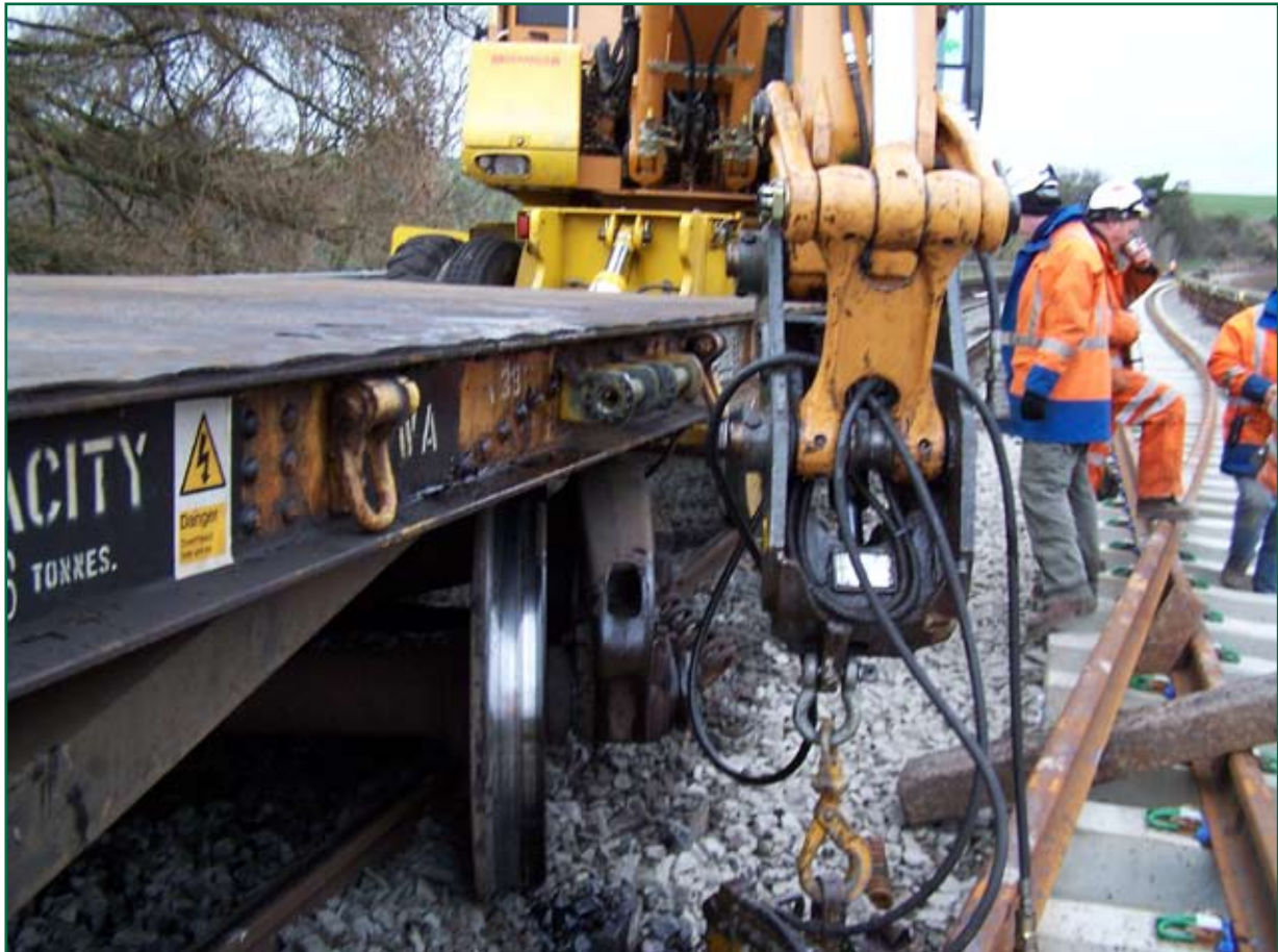
Figure 10: Consequences of the collision (by courtesy of Network Rail)
