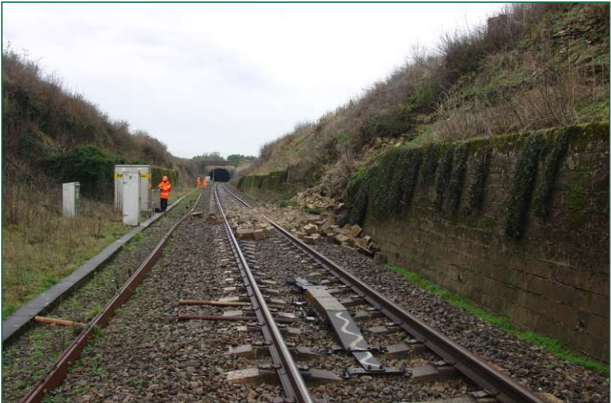
Figure 2: View of derailment site in the direction of travel
