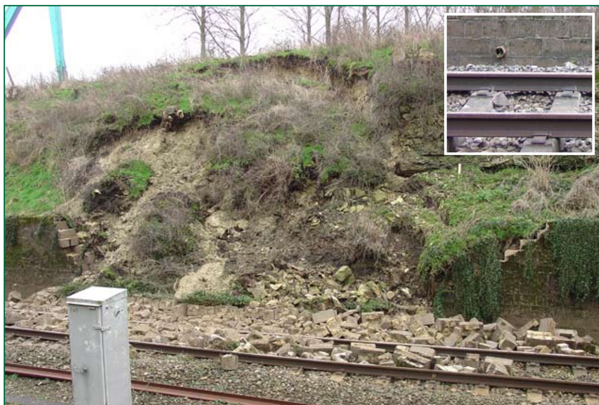
Figure 4: Derailed site showing cutting slips, state of backfill and typical weep hole (inset)
