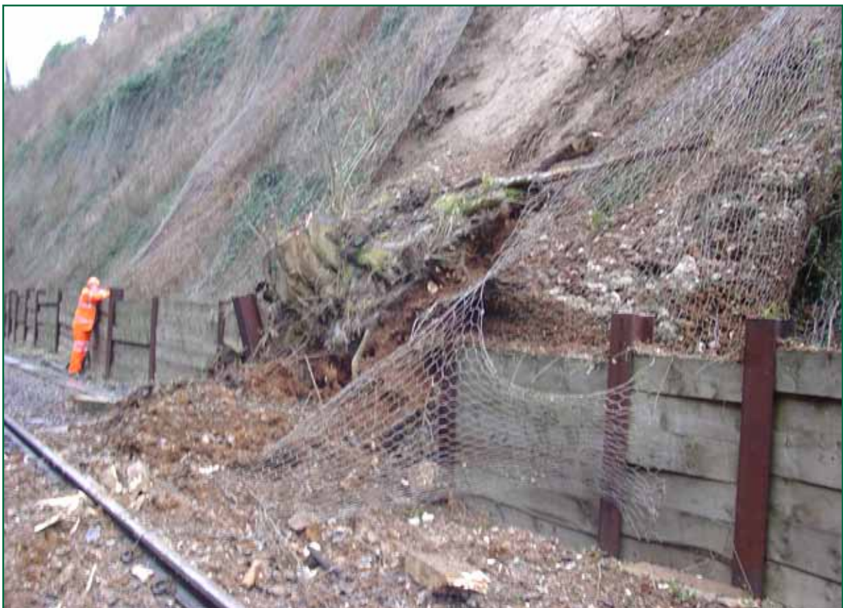
Figure 12: Debris and rootball against the king post wall
