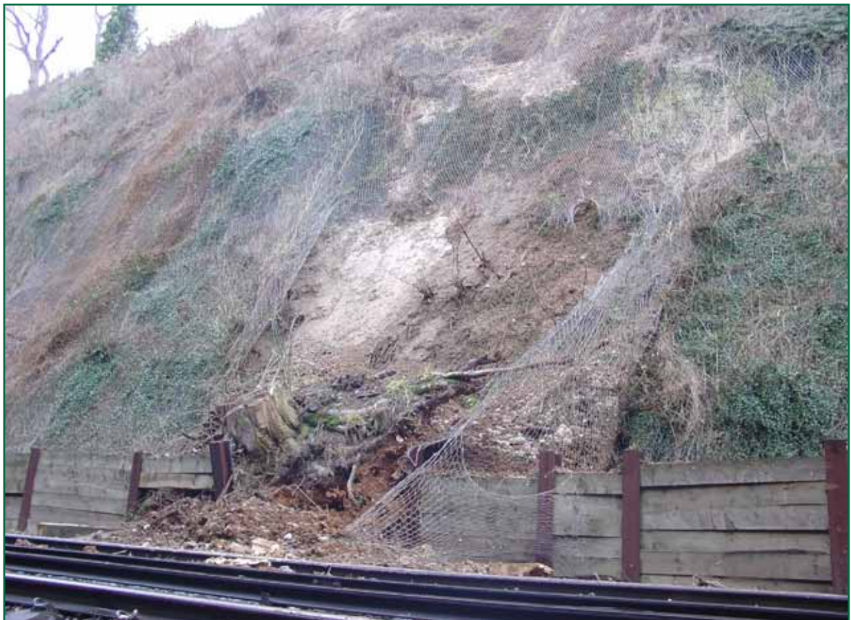
Figure 9: Hooley cutting showing the landslide
