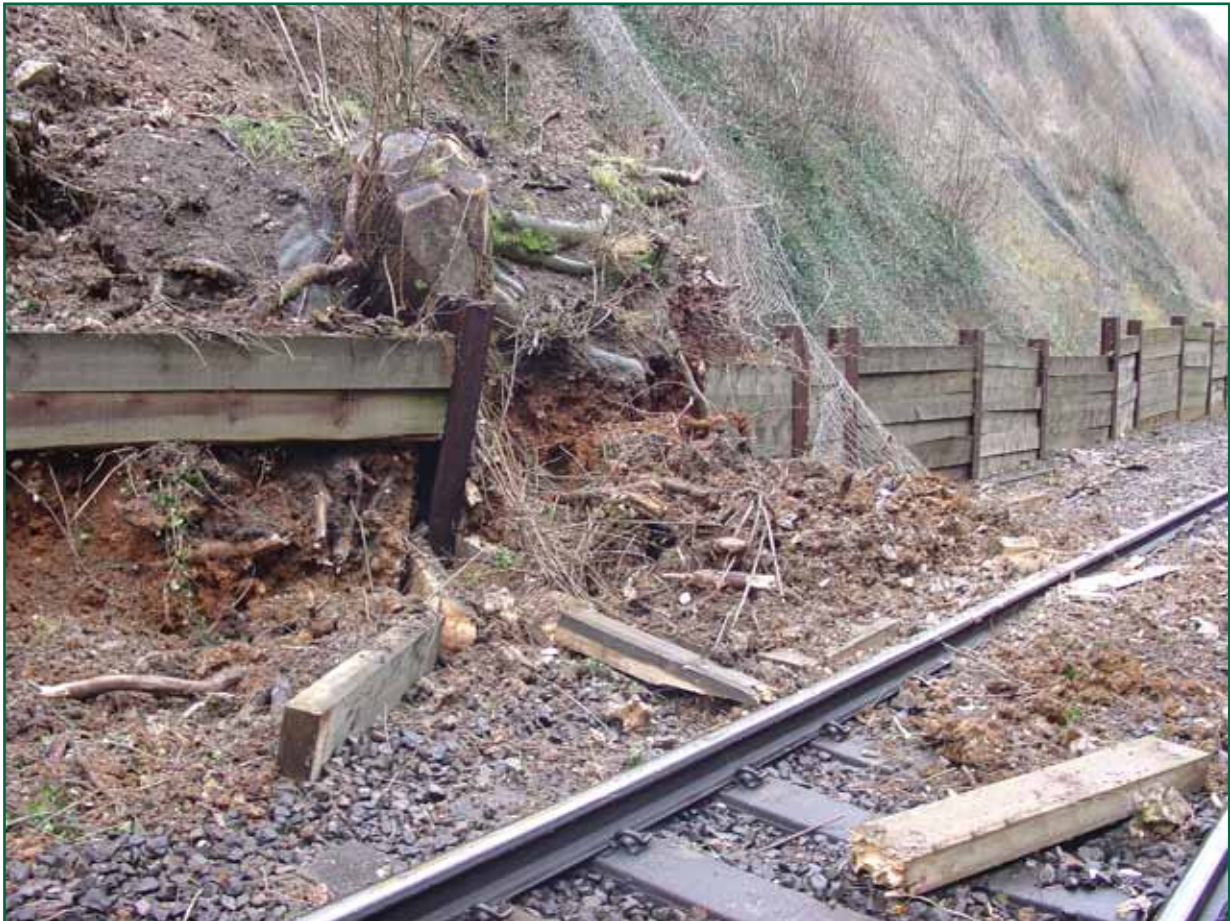
Figure 11: Debris on the track following the derailment
