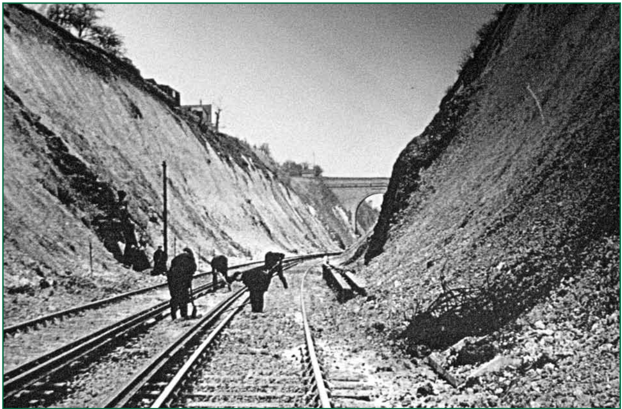
Figure 5: A rock fall on the down side of Hooley cutting during the snows of 1947. The variable depth of gravel can easily be seen on the left side of the cutting (courtesy of Network Rail)
