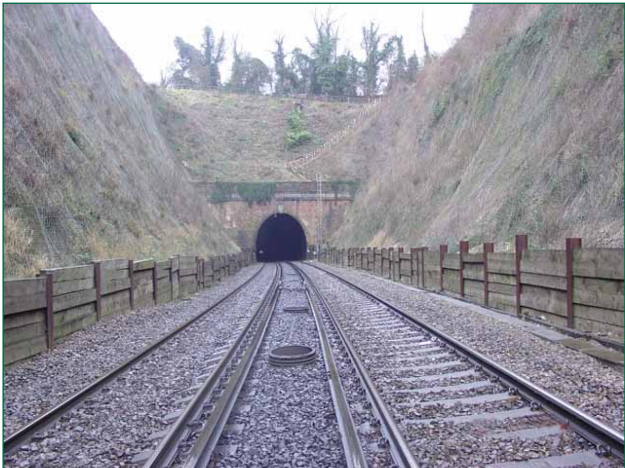
Figure 7: Hooley cutting viewed from the site of the derailment looking towards the tunnel mouth.
