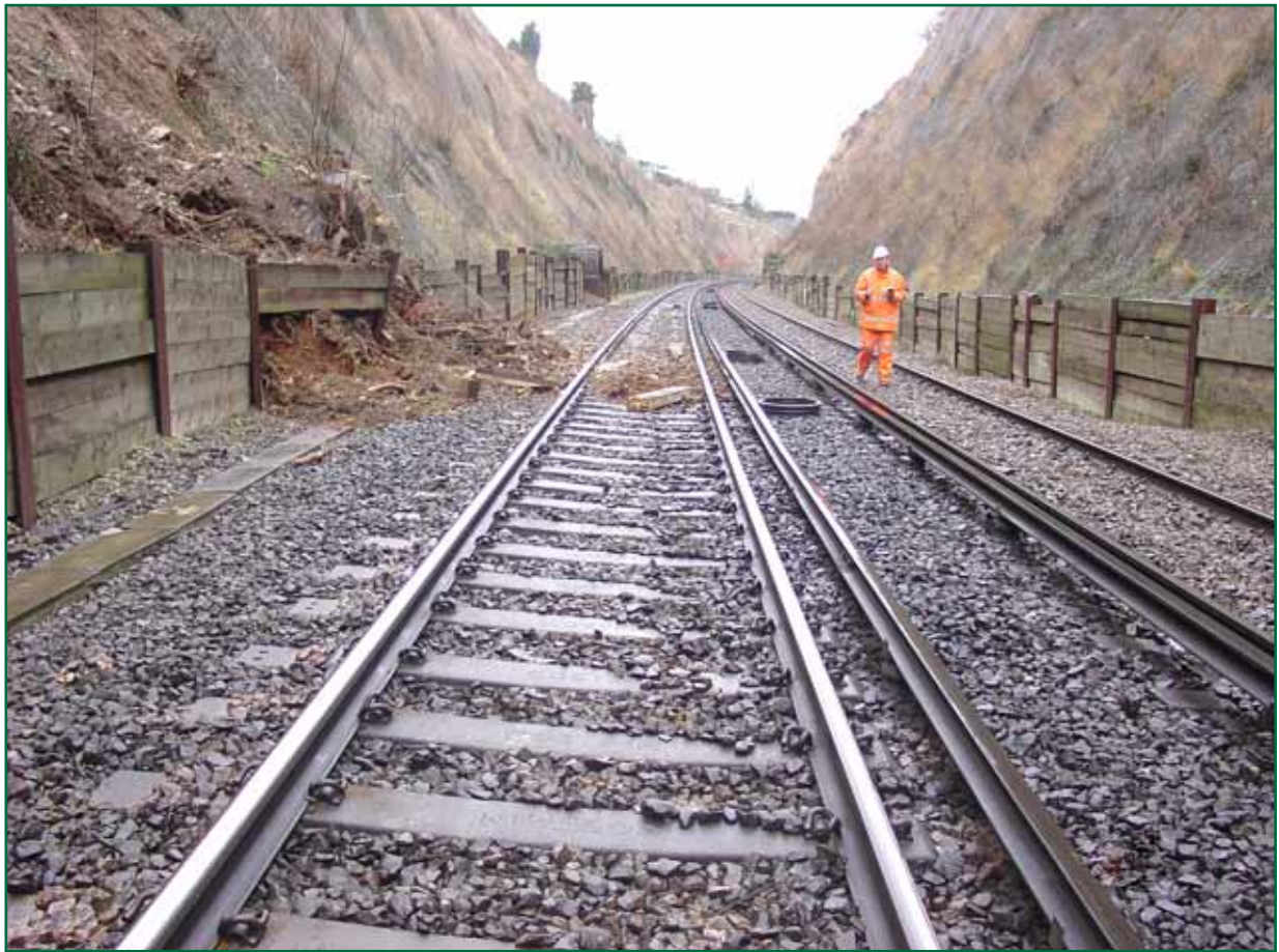
Figure 8: Hooley cutting following the derailment showing the king post wall viewed looking towards London.
