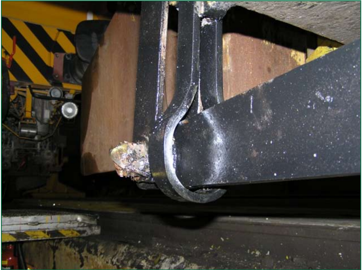
Figure 19: USP 3000 ballast regulator torque arm with recommended safety keep. Similar safety keeps have been fitted to all NIR OTP
