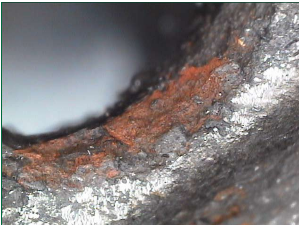
Figure 17: Microscopic image (100x magnification ) of split pin hole. Residual geological debris inside the hole and oxidisation indicate split pin has not been in place for some time prior to the incident
