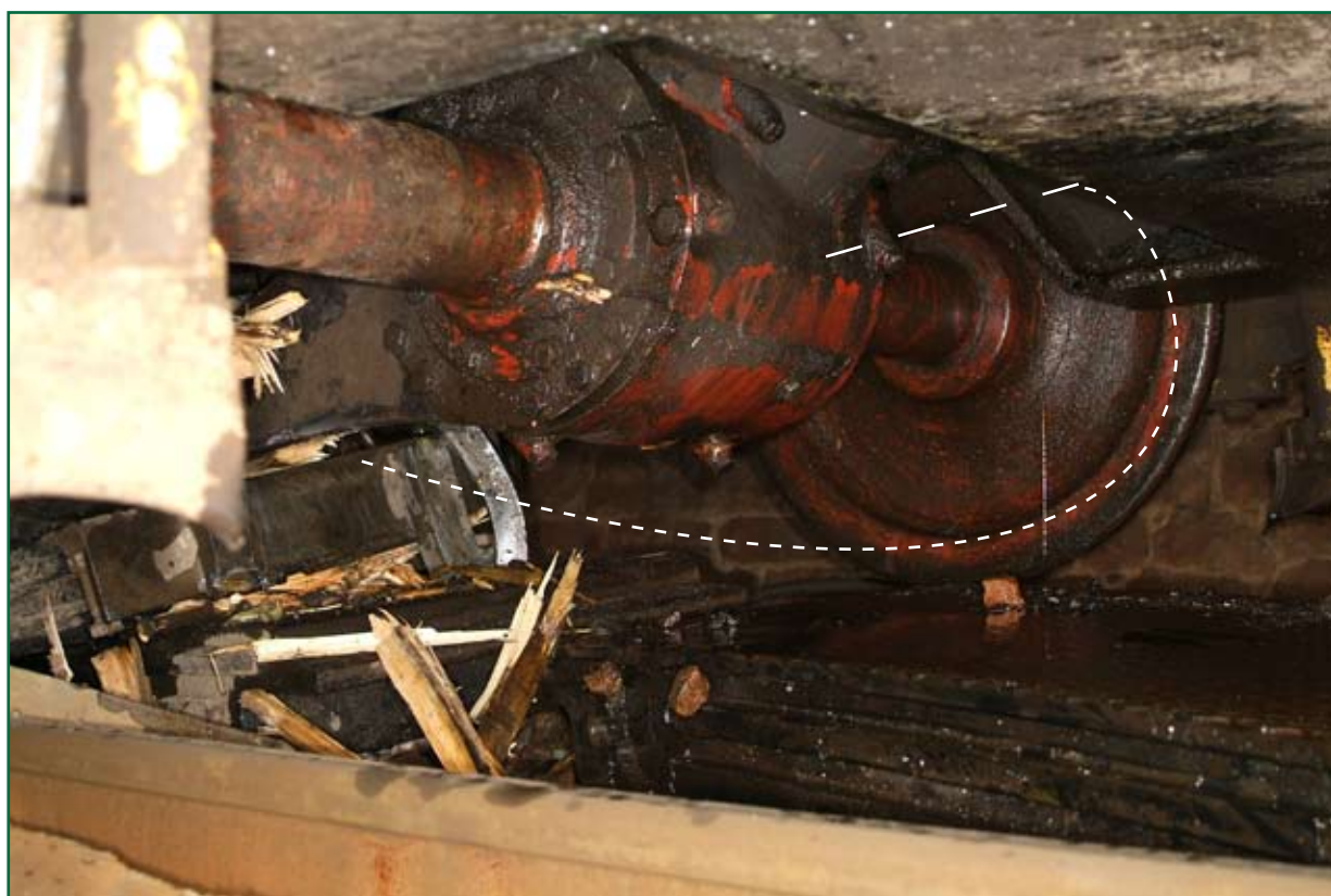
Figure 11: Torque arm damage seen when regulator lifted on site
