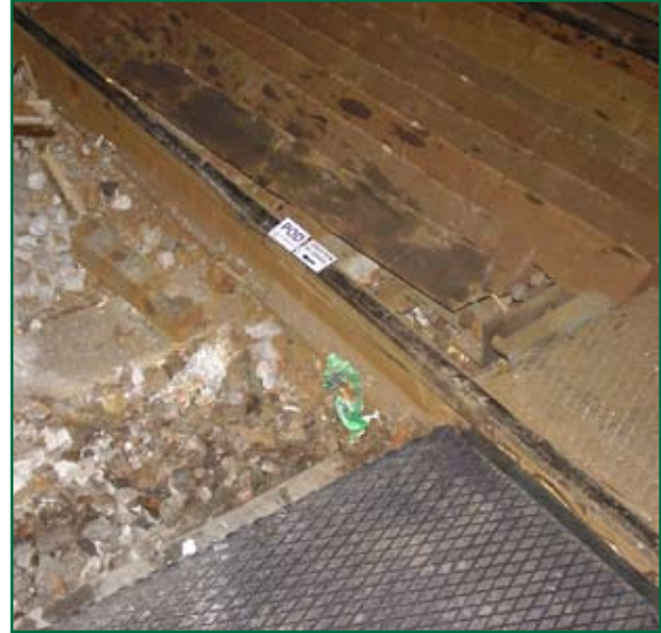
Figure 4a: Point of Derailment (POD) showing sleeper zero
