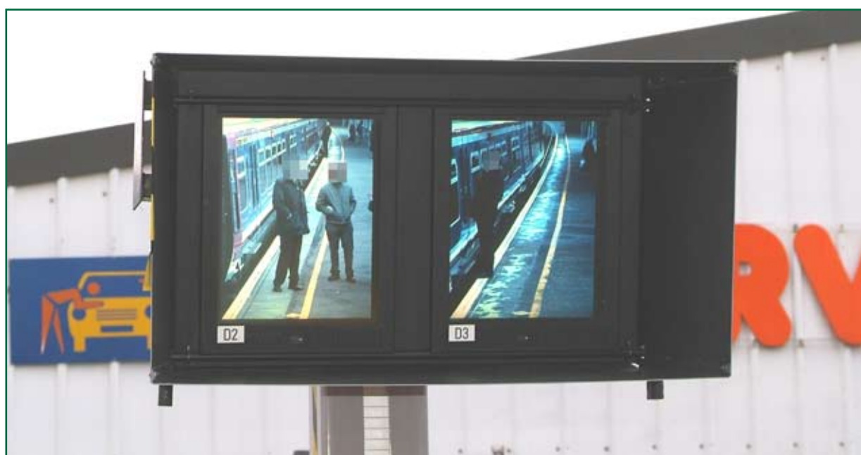
Figure 23: Four-car monitor bank with a Class 365 Unit at a stand taken before the centre-line
