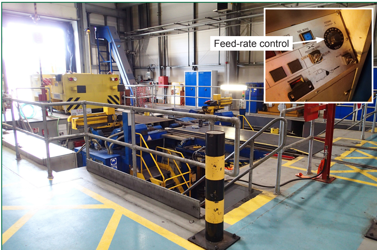
Figure 12: Wheel lathe at Ardwick depot (inset shows the control used to manually set the feed rate on the finishing cut)
