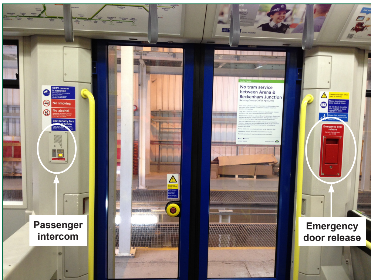
Figure 7: Passenger intercom and emergency door release
