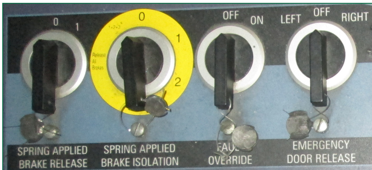
Figure 5: Fault override and brake isolation switches
