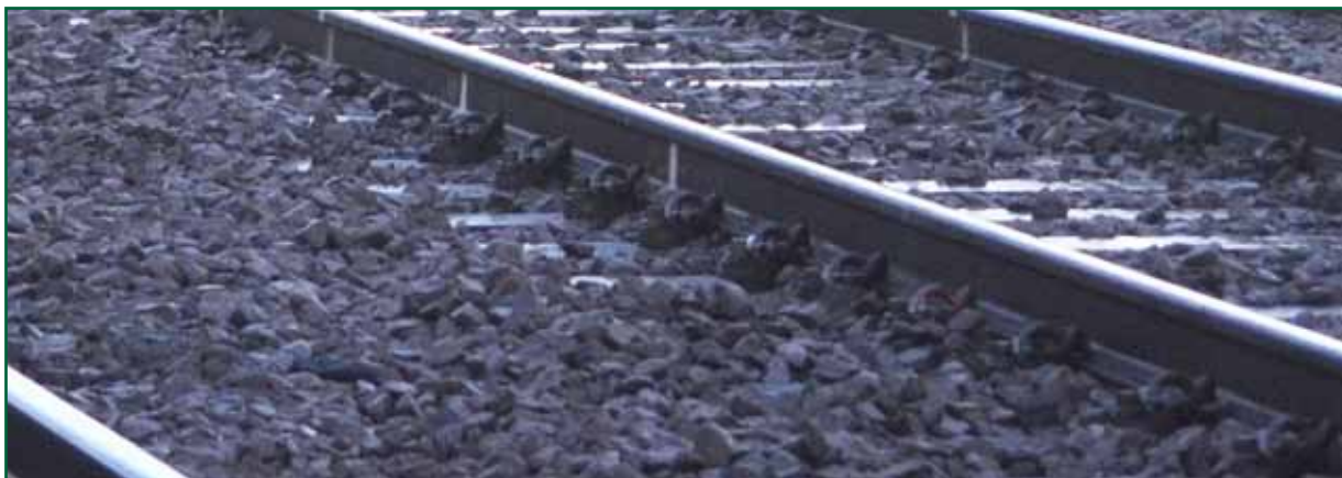
Figure 12: The scene of the accident looking at the area of work on the down line with ballast tidied around the sleeper ends within the six-foot
