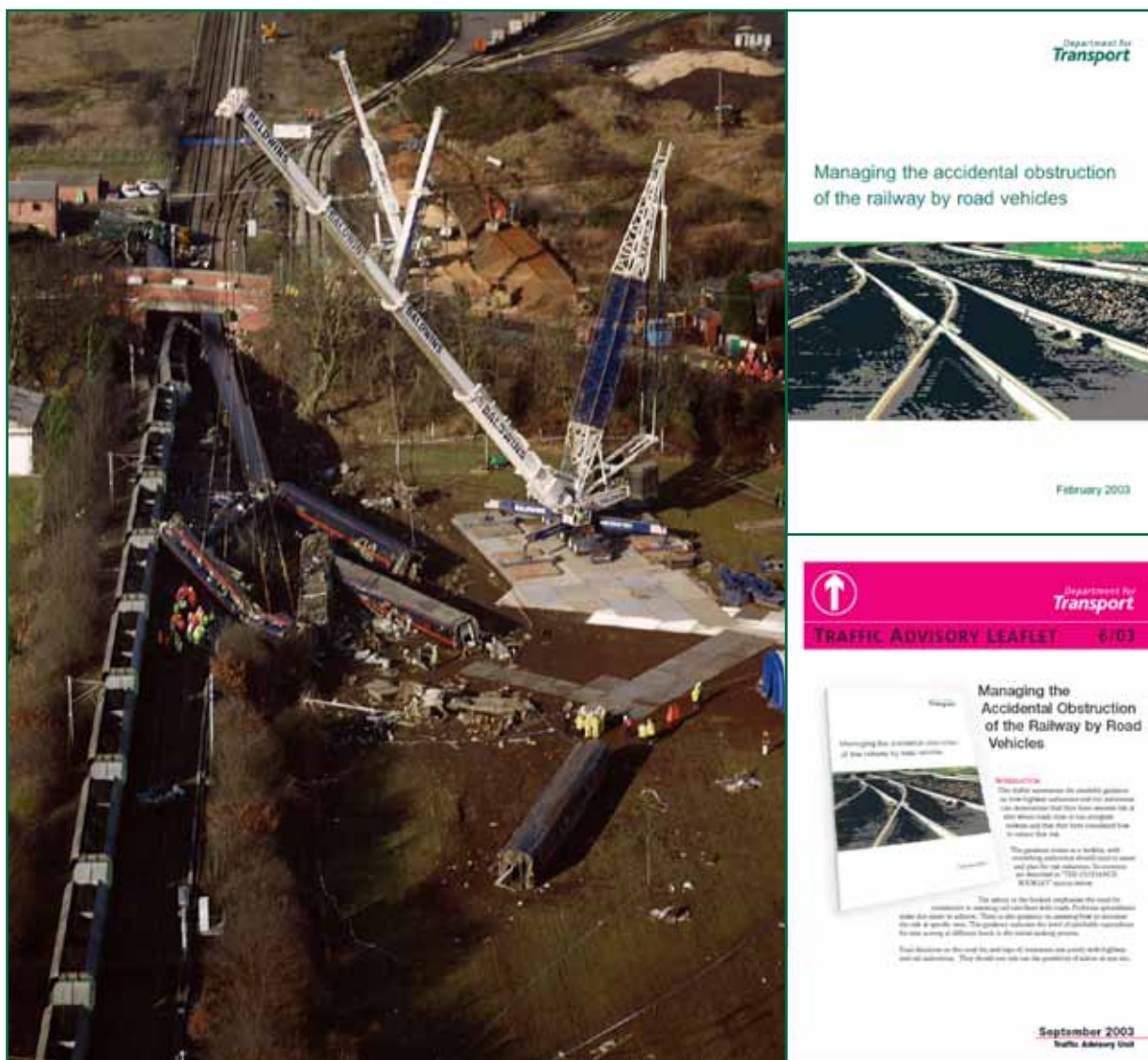
Figure 5a: The Great Heck accident (left); 5b (above right) DfT guidance document; and 5c (bottom right) traffic advisory leaflet sent to all local authorities in 2003. Both documents outlined the process and requirements for RVI assessments.
