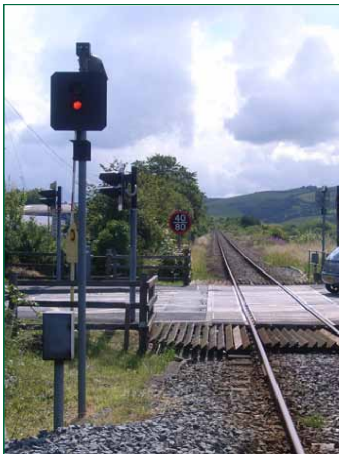
Figure 6: Llanbadarn ABCL showing driver's crossing indicator (DCI) flashing red
