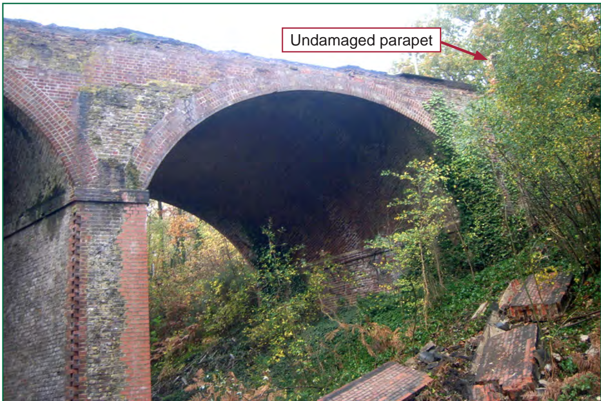
Figure 13: View of bridge and missing parapet from track level. The parapet fell in sections weighing up to 1800 kg
