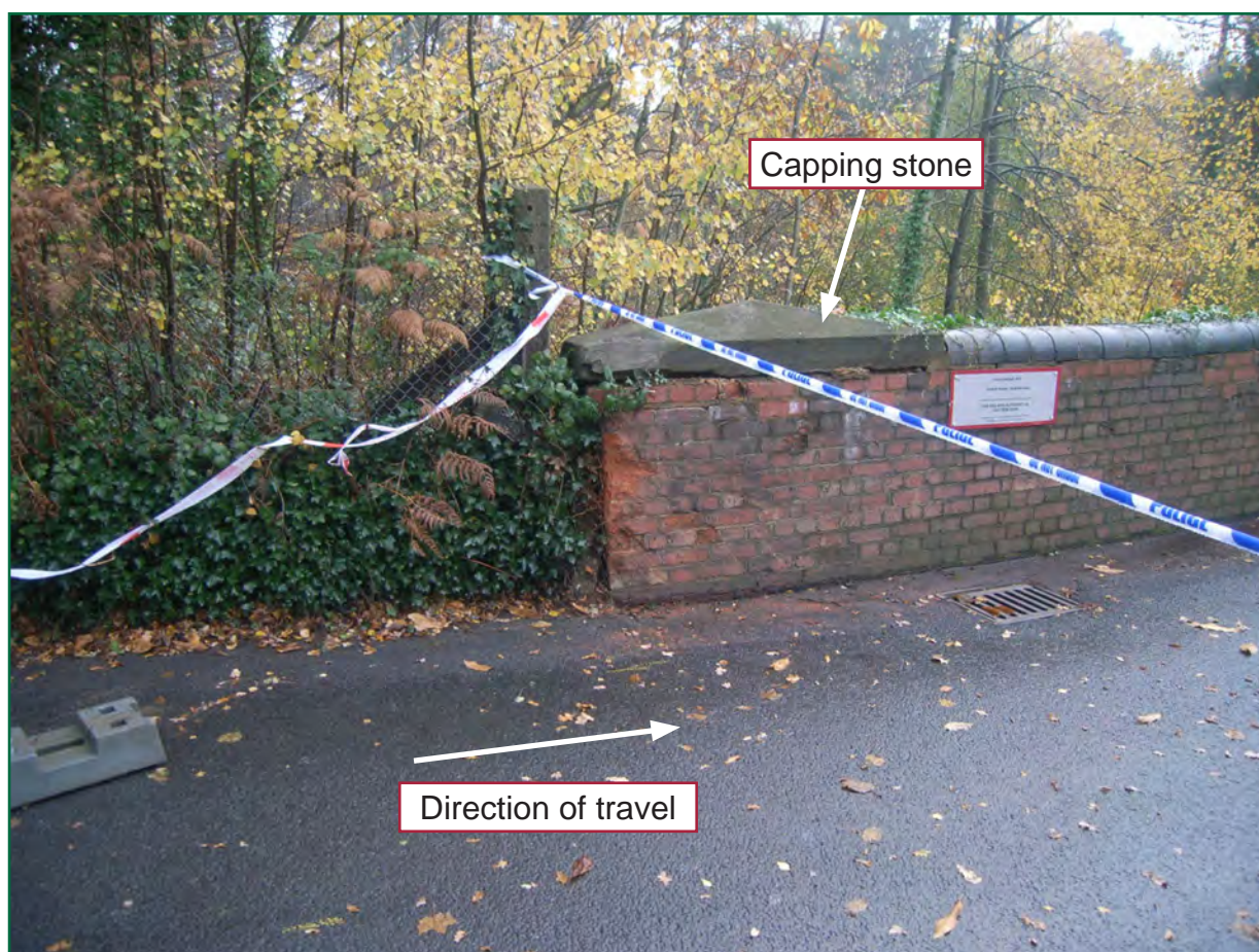
Figure 4: North end of the east parapet which was struck by the lorry
