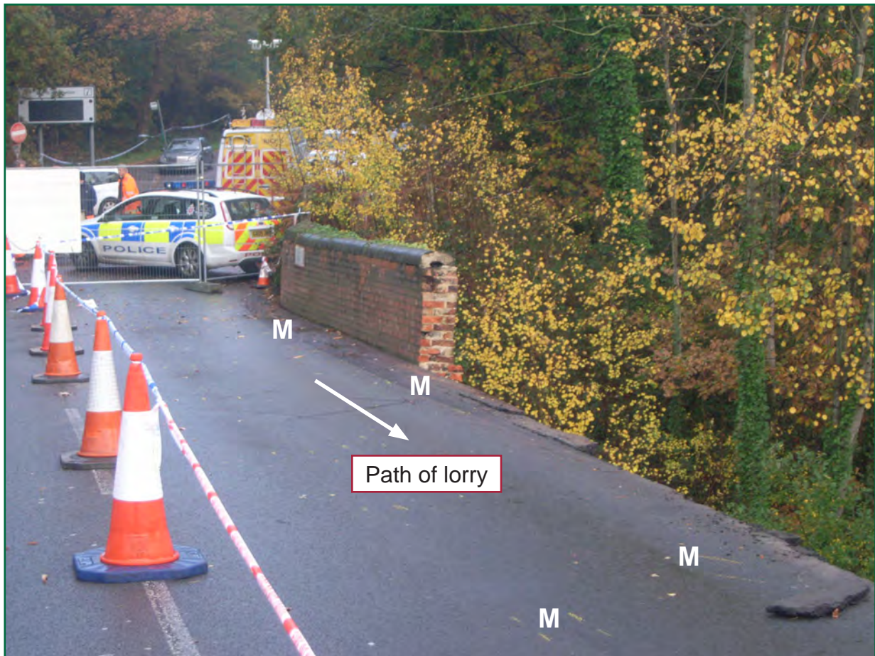
Figure 5: Photograph of bridge deck showing missing section of parapet and skid marks denoted 'M'
