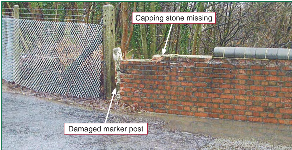
Figure 10: Photograph of the north end of the east parapet showing 'new and longstanding damage' after a similar collision in December 2003 (photograph January 2004, courtesy of Network Rail)
