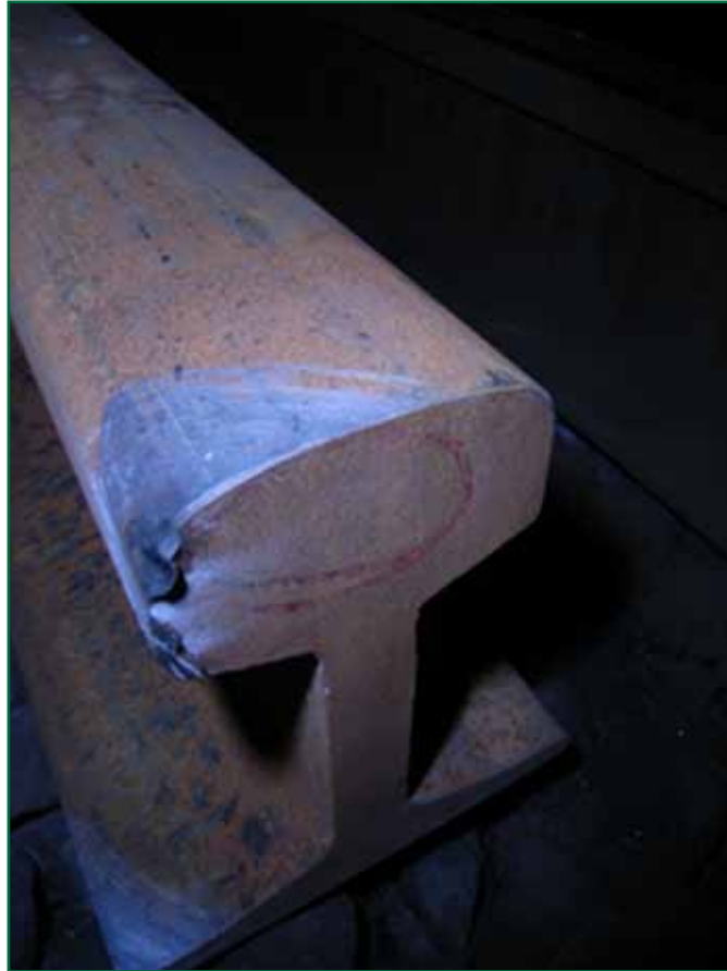
Figure 5: Damaged rail end
