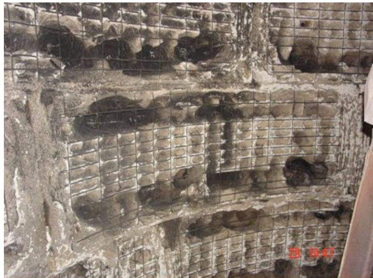
Figure 35: Damage suffered by the tunnel lining at the level of the tunnel roof
