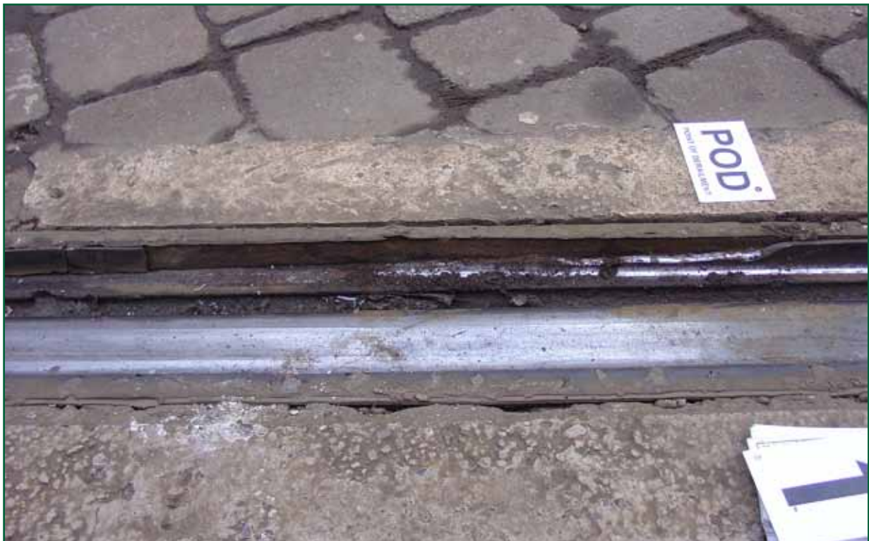
Figure 4: The right-hand rail at the point of derailment where the keep had failed
