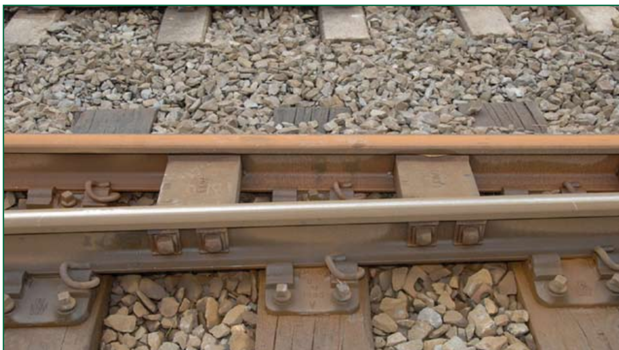
Figure 5: Cast iron blocks joining switch and stock rails
