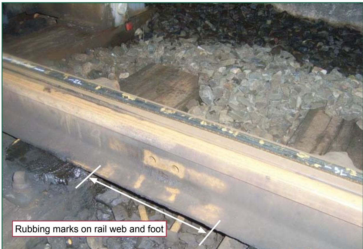
Figure 19: Marks on rails showing limits of movement of second stretcher bar
