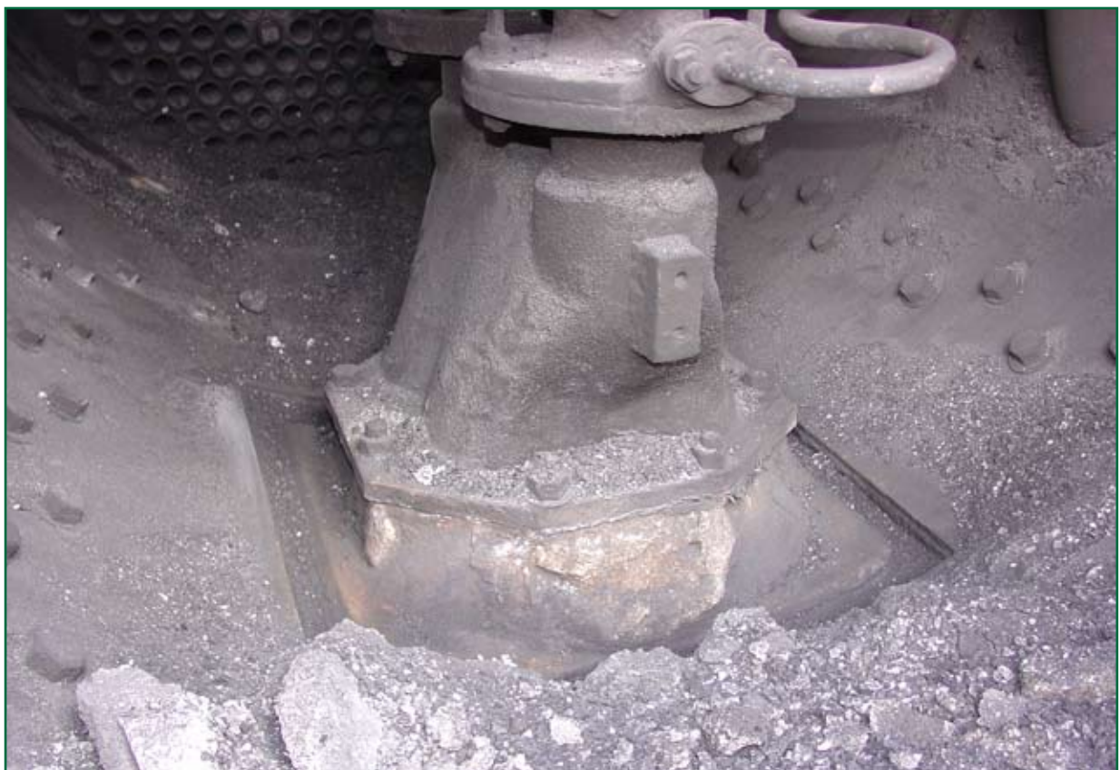
Figure 8: The blastpipe in-situ
