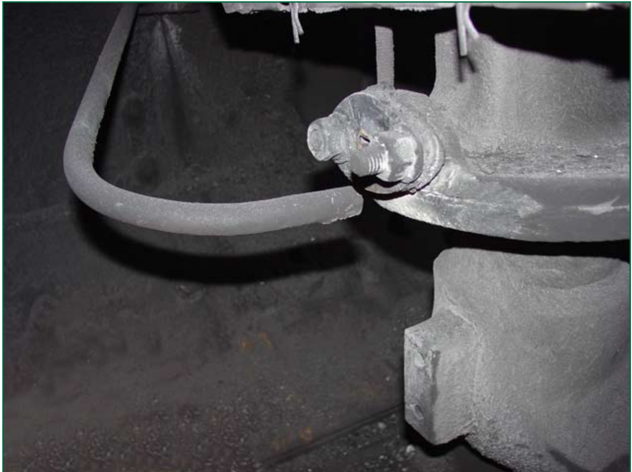
Figure 7: The fractured rear blower feed pipe in-situ
