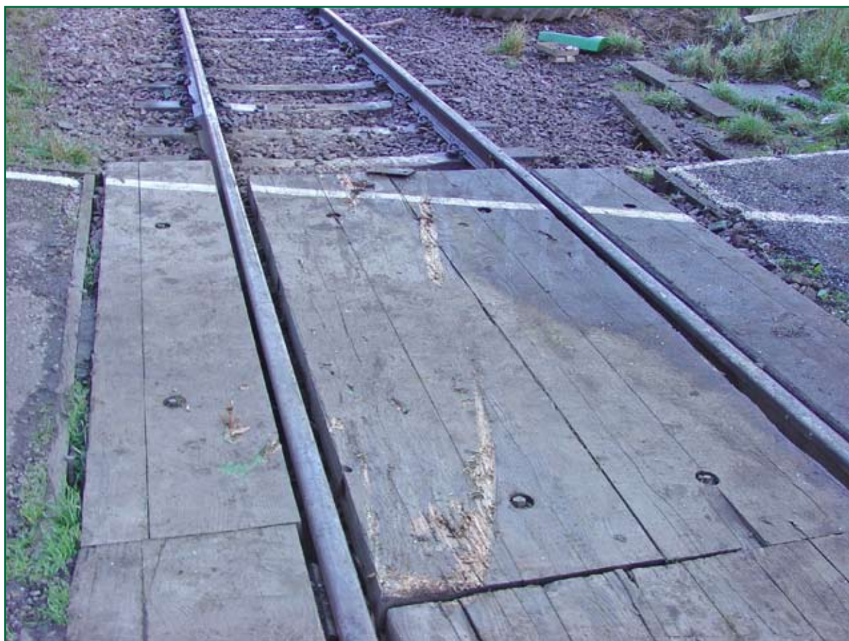
Figure 8: Gouge marks on crossing surface
