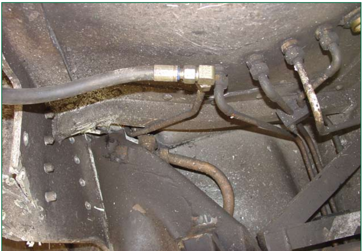
Figure 14: Buckled floor plate beneath train cab
